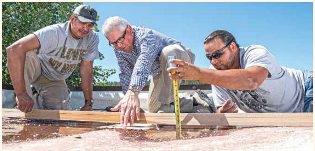
Brian Red Star, Mike Skaggs and Rich Miner inspect the collapsing, leaking roof above the kitchen.
