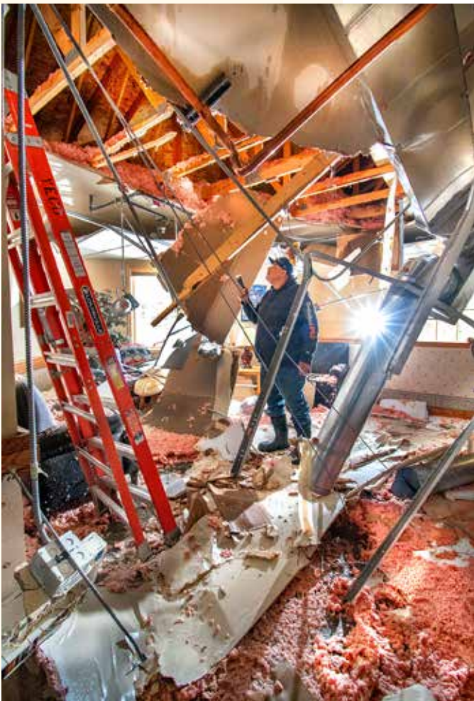
Inspecting the catastrophic damage from broken pipes.
